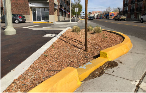
A curb cut to a bioswale allows stormwater to infiltrate through the soil naturally instead of being directly diverted to storm drains, Albuquerque, NM
